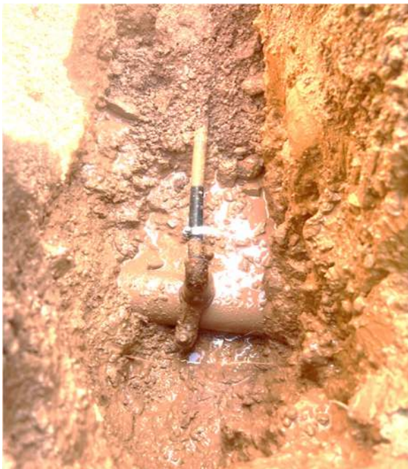
Leaking Service line incorrect Installation
